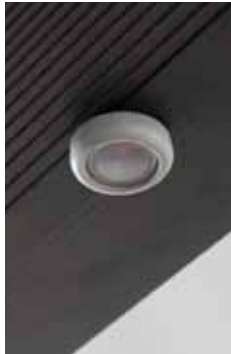
Detail photo of controls
